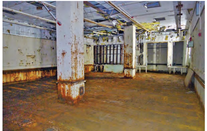
Present day photo of Tape Handler room. Note the damage to the ceiling and rear wall caused by FAA bomb hardening testing after site closure
